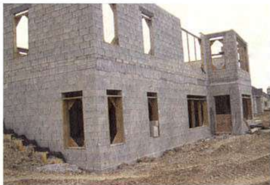
This rear view of David & Goliath Builders, Inc. Cobblestone Ranch model shows the concrete-block construction.
